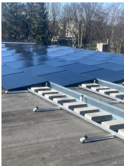
Solar Panels on Roof
