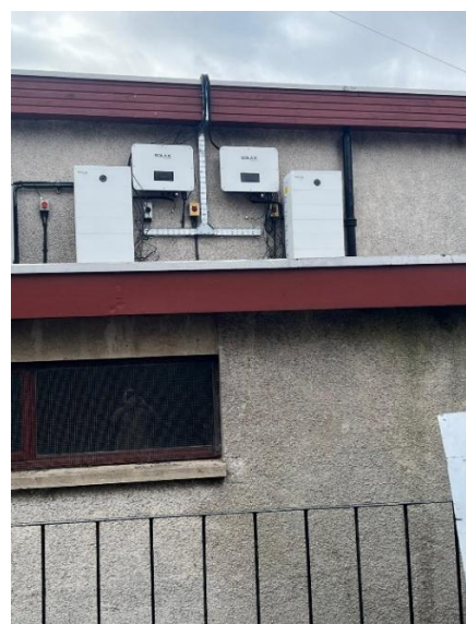
Battery Backup Units & Inverters
