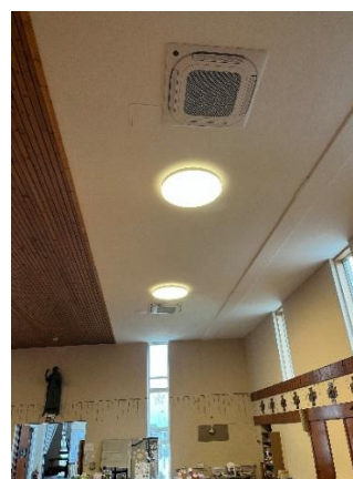
Inside unit beside lighting
